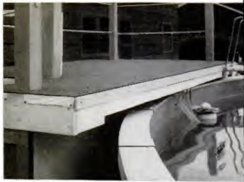
PLATFORM OVERHANGS pool slightly; measurements might vary from drawing to suit different size pool
